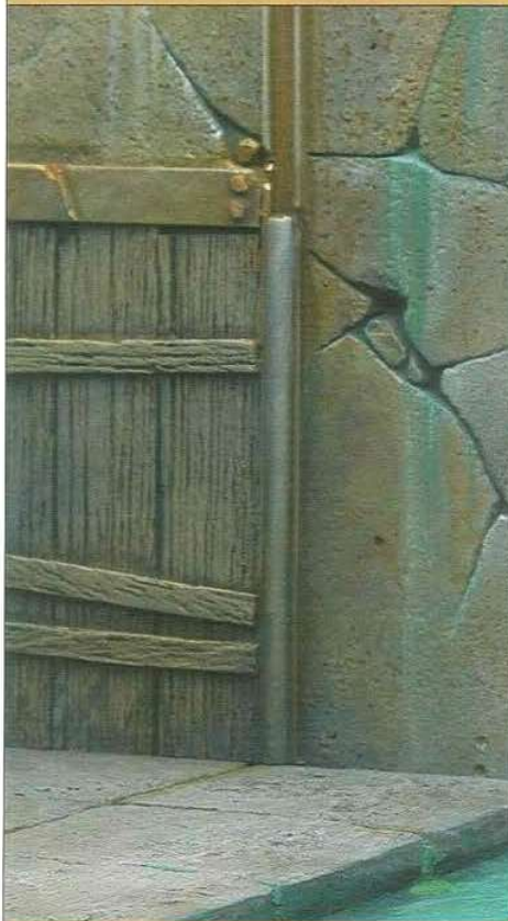
THE WALLS SOMETIMES TRICKLE WITH WATER DUE TO THE GROUND WATER NEARBY.
